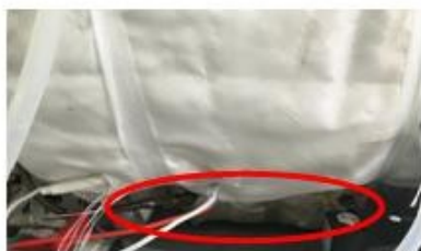
Sealed steam generator
