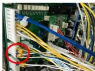
Wire line of outer sensor 3#
