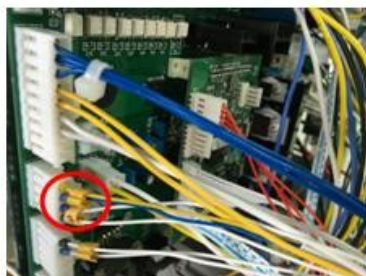
Temperature sensor of steam generator 1#
